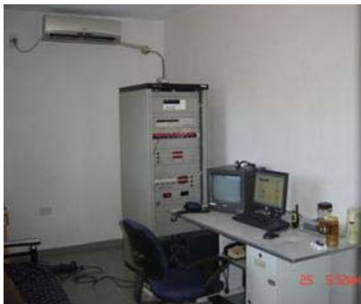
Figure 8: Control Room for SLR
